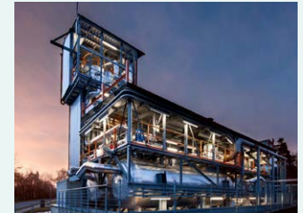
Thermal energy storage TESIS Photo: DLR (CC-BY 3.0)
